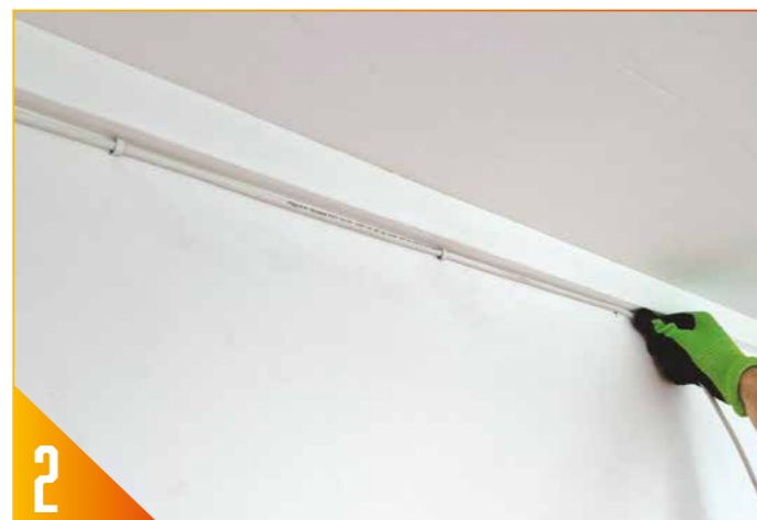
2 Drill the required holes for all FireClips and push clips over the RTRYVA cable to fix into place.
