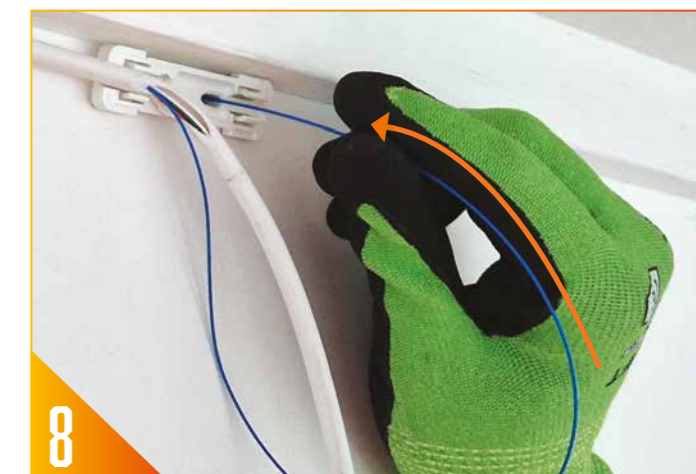
8 Once the fibre has been retracted, start pushing it through the drop tube to the other side of the wall into another Break-Out Bend Manager.
