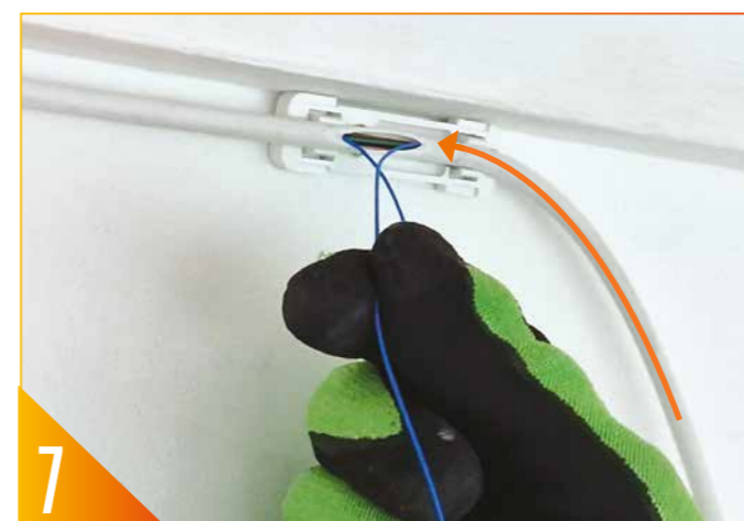
7 Place the cable back into the Break-Out Bend Manager, now the fibre can be selected and pulled back.
