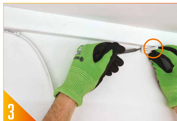
3 Using the Break-Out Bend Manager, mark out and drill the passage for the fibre drop to the other side of the wall.
